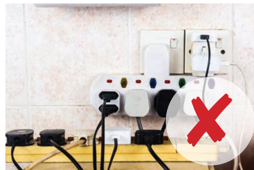
Never overload indoor or outdoor sockets. This could cause a fire.
